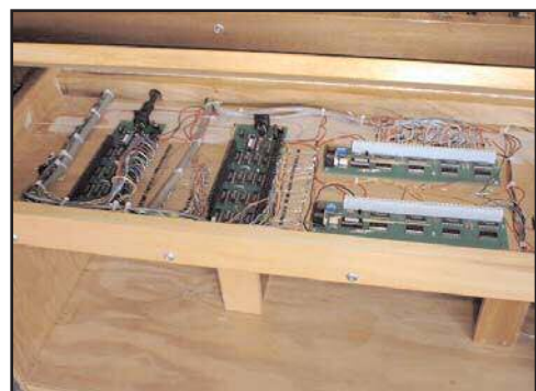
Figure 8. The interface with the MIDI boards on the left and Midiman couplings on the right. The photo was taken before final installation.
